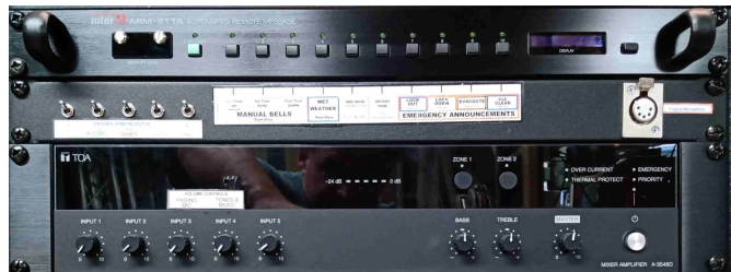
Equipment located in Main Office Compact 4RU Rack
