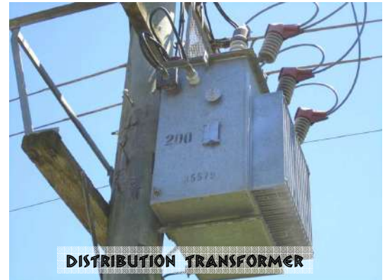
Typical Australian pole transformer . The “200” denotes the capacity—in this case 200kVa, enough power for about 16 typical homes.
